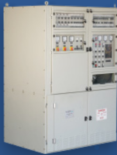
Switch Board Cabinet
