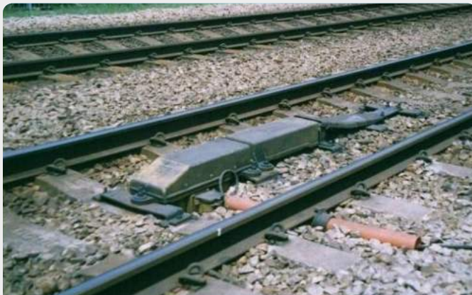
Position of AWS Ramp in the track on the approach to a signal
