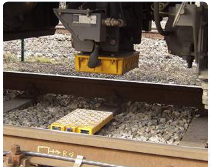
Track Mounted balise and the Train Mounted Data Reader
